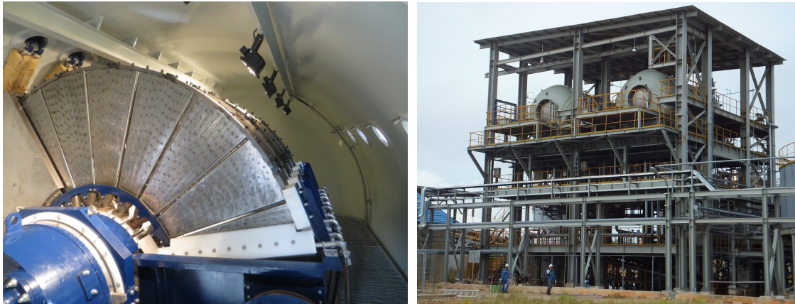
Figure 1: HiBar disc filter (70 m 2 ) with steam cabins in the vessel for steam pressure filtration of bauxite residue (left) and filter building with both units (right)
